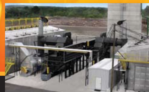
"Saw Mill Converts Waste-to-Energy" Lumber Curing Fuel Cost Reduced
