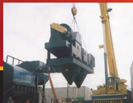
Twin Ash Collectors Primary and Secondary Modular Units Being Lifted in Place.
