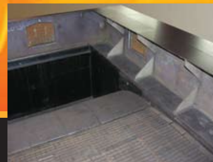
Automated Ash Removal (Wet System)
