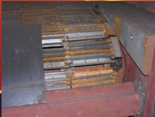
Triple 600 BHP w/ Silo Fuel Storage
